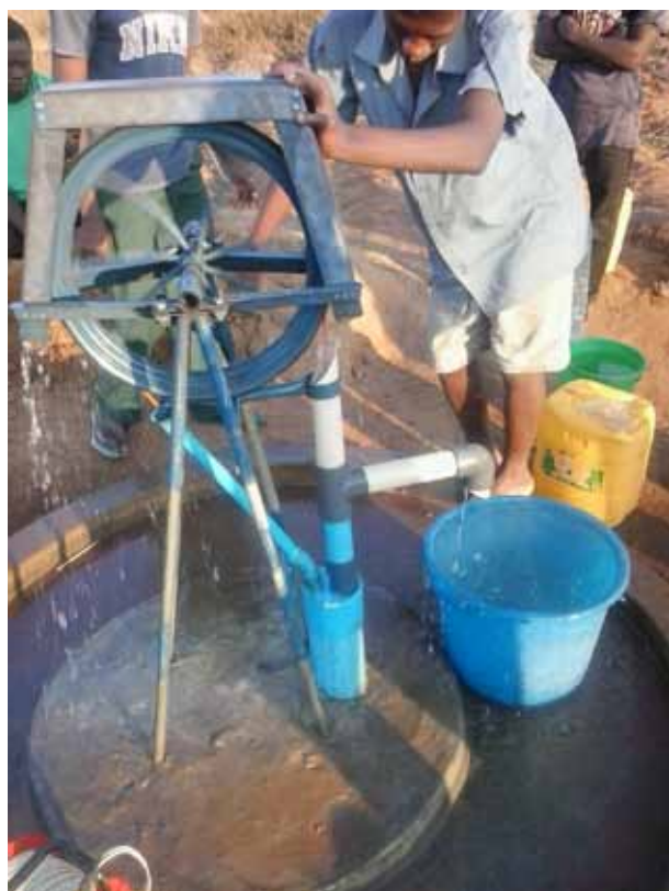
Top photo: Rope pump on the hand drilled tube well of 25 meters deep, including an apron and soak away.
